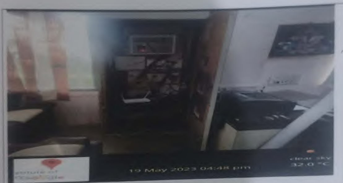
Internet & Router connection panel
